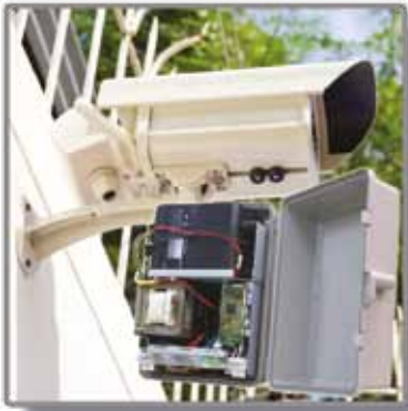
Pole Mounted UPS for CCTV
