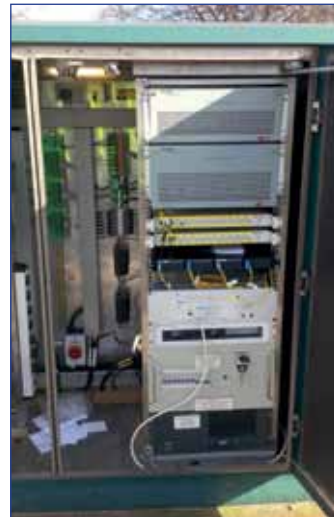
A typical 10 year old system supplied by Harland Simon including integrated maintenance bypass switch and 10 way distribution panel all built into the customer's outdoor enclosure
