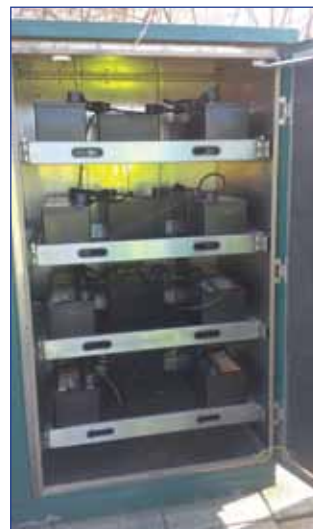
A typical 3 hour autonomy battery arrangement in outdoor enclosure with additional battery charger modules enabling batteries to be re-charged within 12 hours
